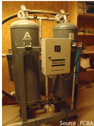
Air "drier" for compressed air compressor
