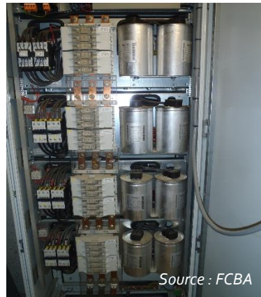
Capacitor bank for a canter line
