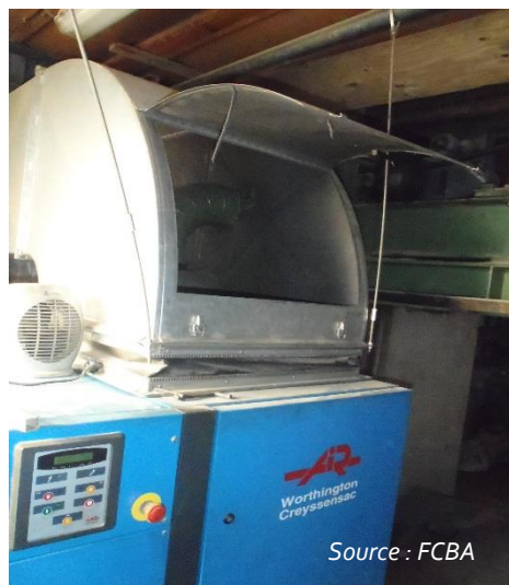
Heat exchange system for the compressor
