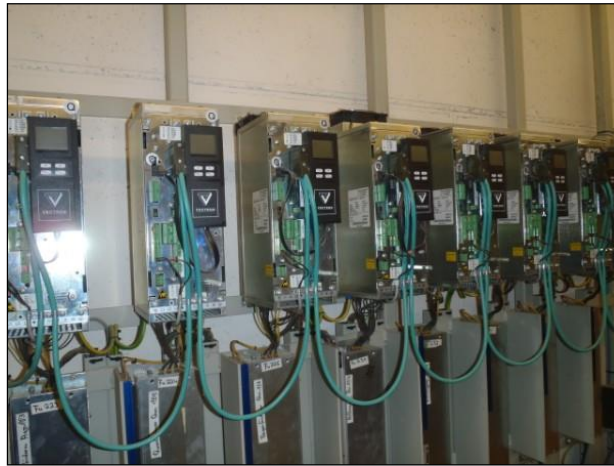
Variable frequency drives for production machinery
